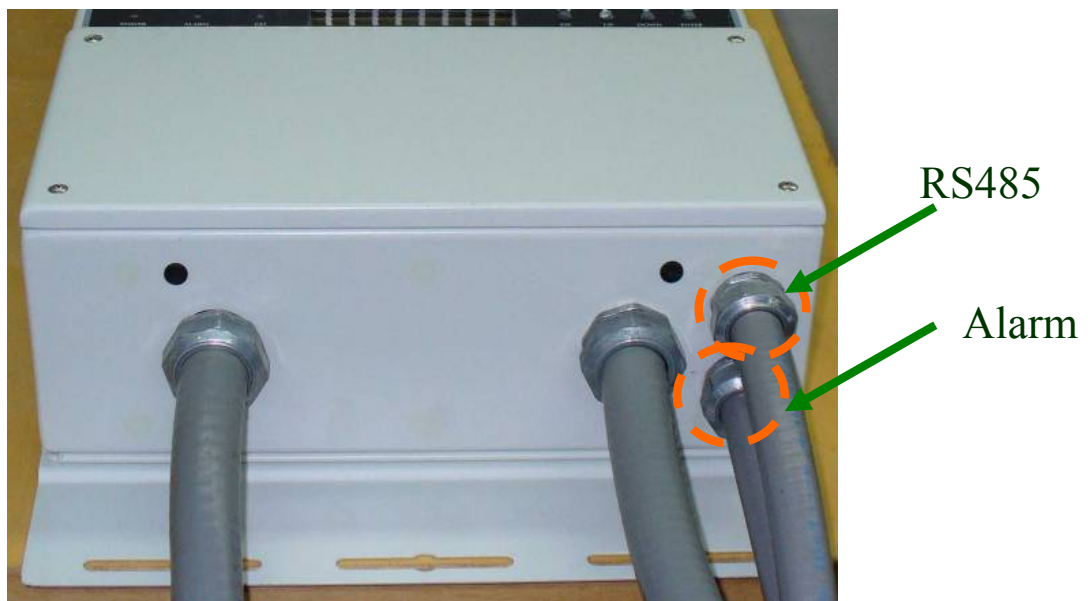
Fig.23 - Hole for cables necessary for RS-485 port connection or wiring for RJ12 connectors connection.
