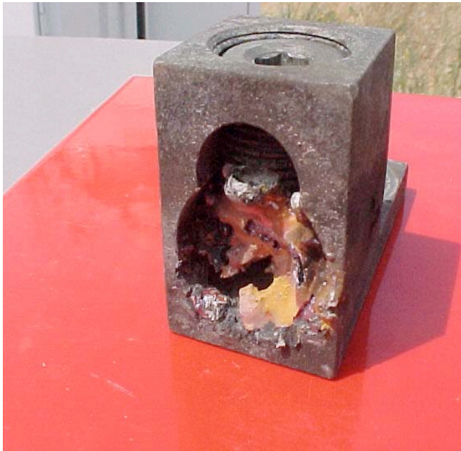
Figure K-2. Destroyed Mechanical Terminal From PV System
