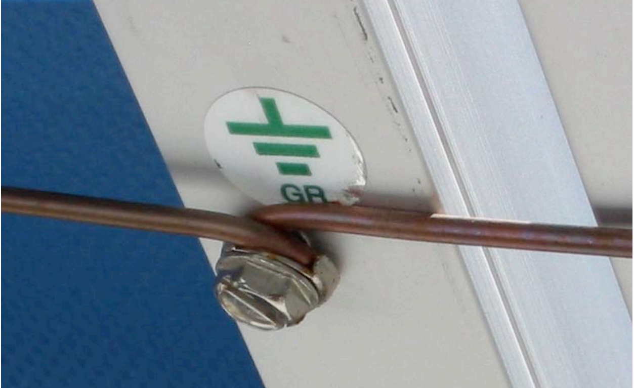
Figure G-2. Improper Module Grounding
